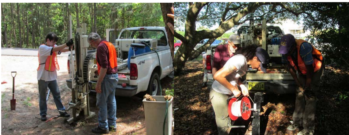
Figure 5 Well installation using a 'geoprobe' drilling rig and recording the depth to the groundwater level in a monitoring well using a water level meter.
