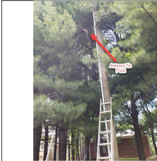
Figure 13a: Power Pole with Antenna
