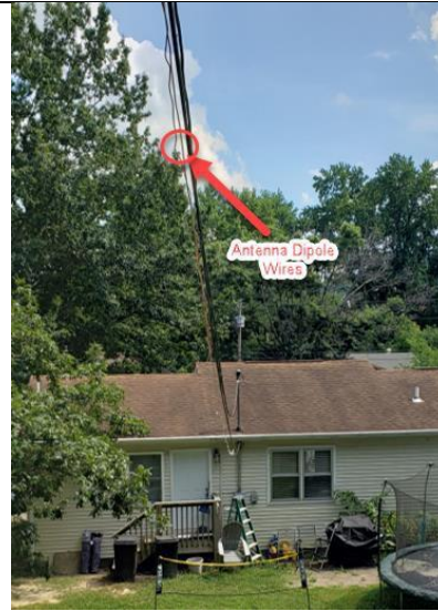
Figure 13b: View of Antenna from Power Pole
