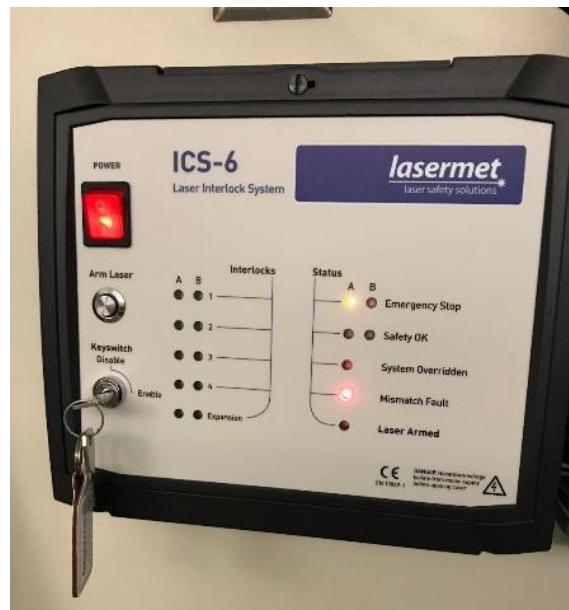
Fig. G.2 The laser interlock system board ICS 6.
